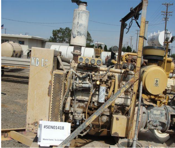
Marioni Project #1 (Old Engine)
