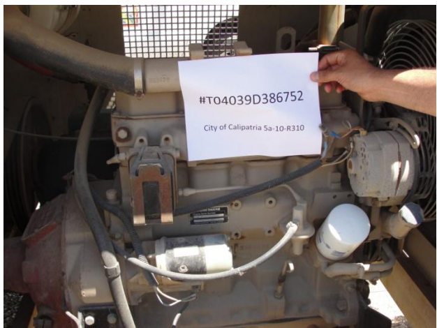
Calipatria Old Sewer Jet Cleaning Pump
