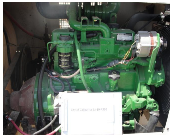
Calipatria New Sewer Jet Cleaning Pump
