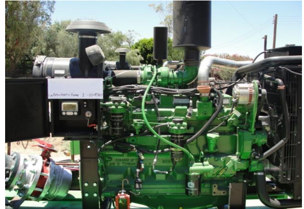
New Agricultural Water Pump Engine at La Brucherie Farms
