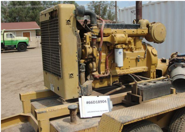
La Brucherie Project #1 (Old Engine)
